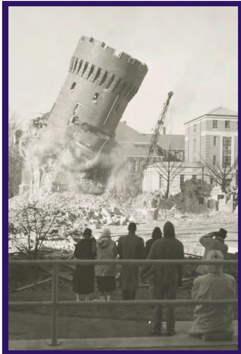
Demolition of the Ohio State Armory and Gymnasium in 1959. Photo courtesy of The Ohio State University Archives.
